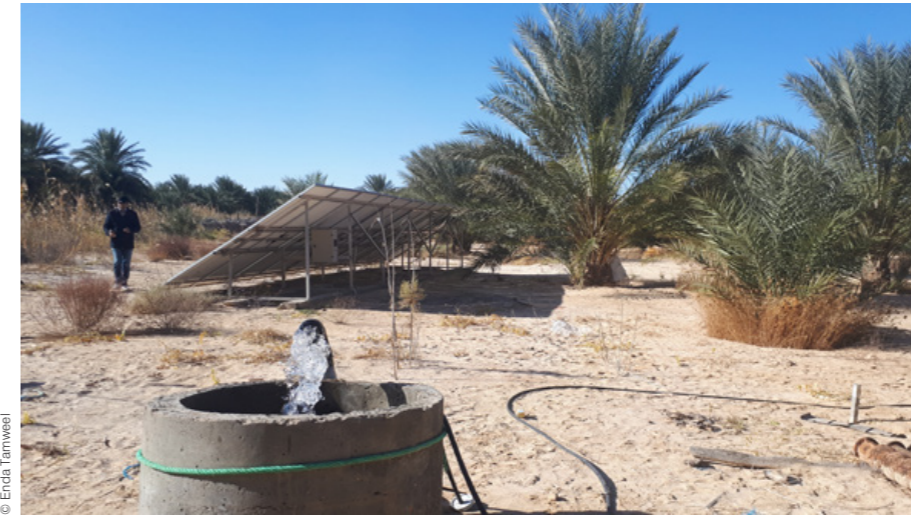
The irrigation system is operated with photovoltaic panels. The pump draws groundwater with energy generated by these panels.
